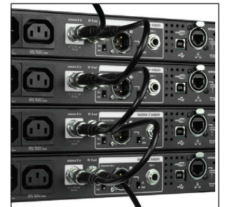
RF distribution ports allow up to 10 receivers to share a single pair of antennas.
